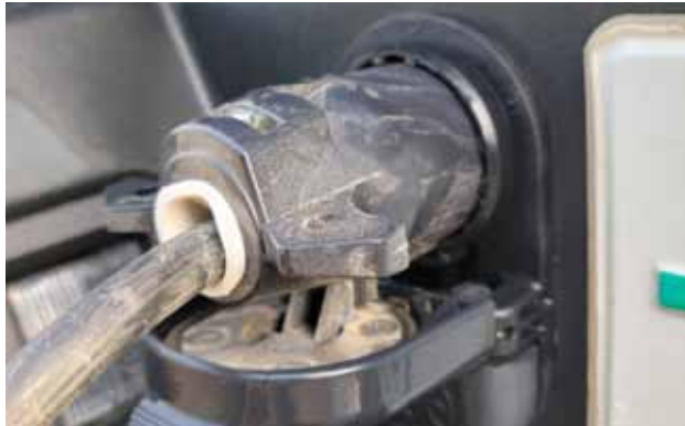
Wiring Harness - Connected
