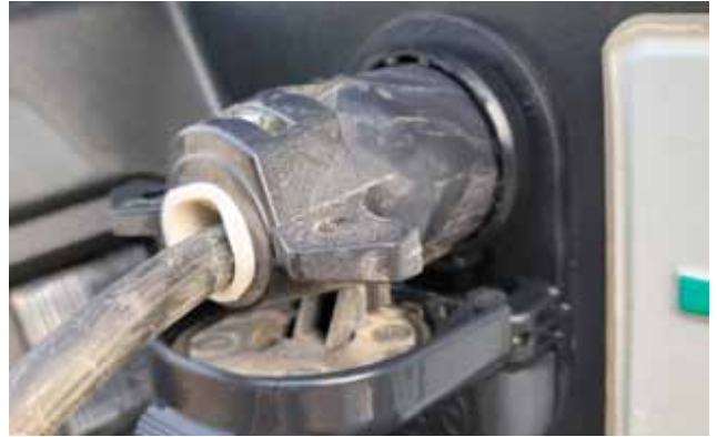
Wiring Harness - Connected
