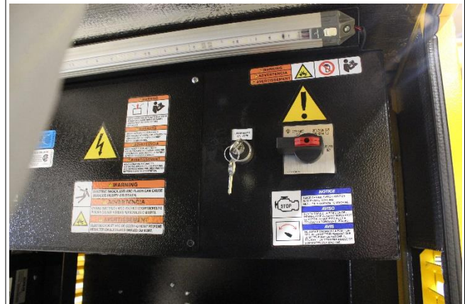
Load Bank (Typical)
