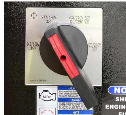
Voltage Selector Switch
